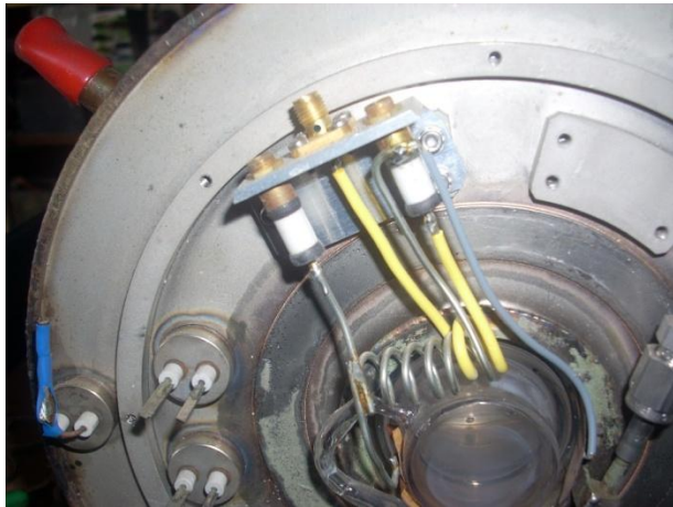
Disassociator RF wiring
